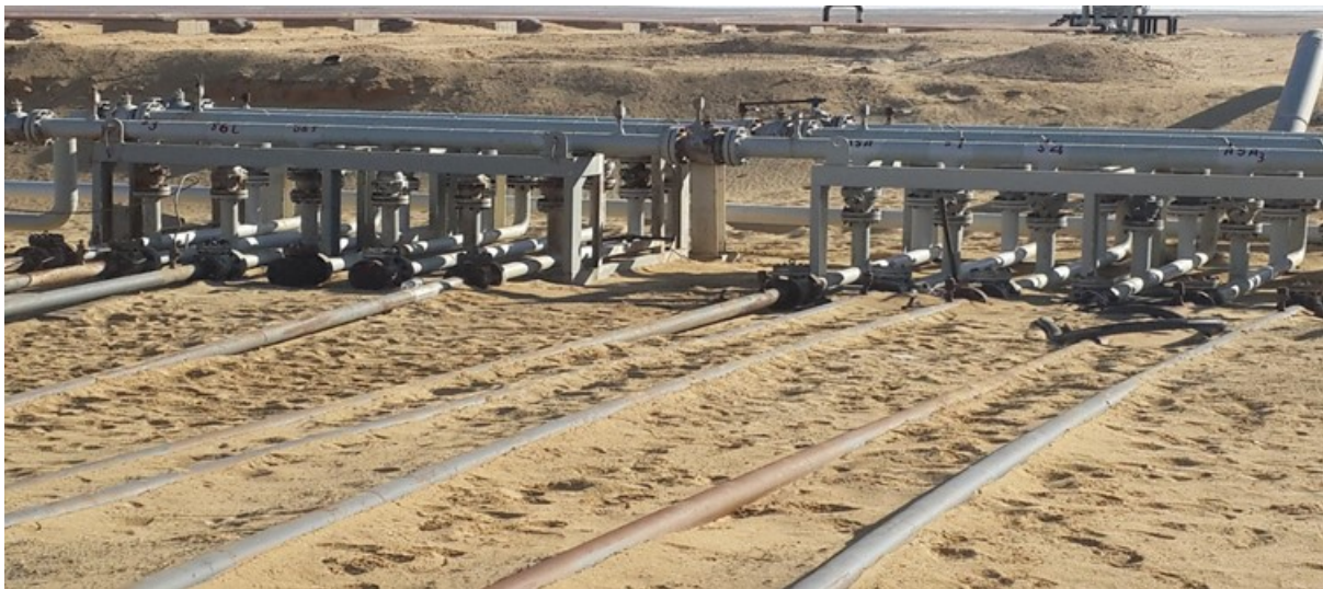
Figure AIV.2: Production Manifold at El Salmiya Oil Station
