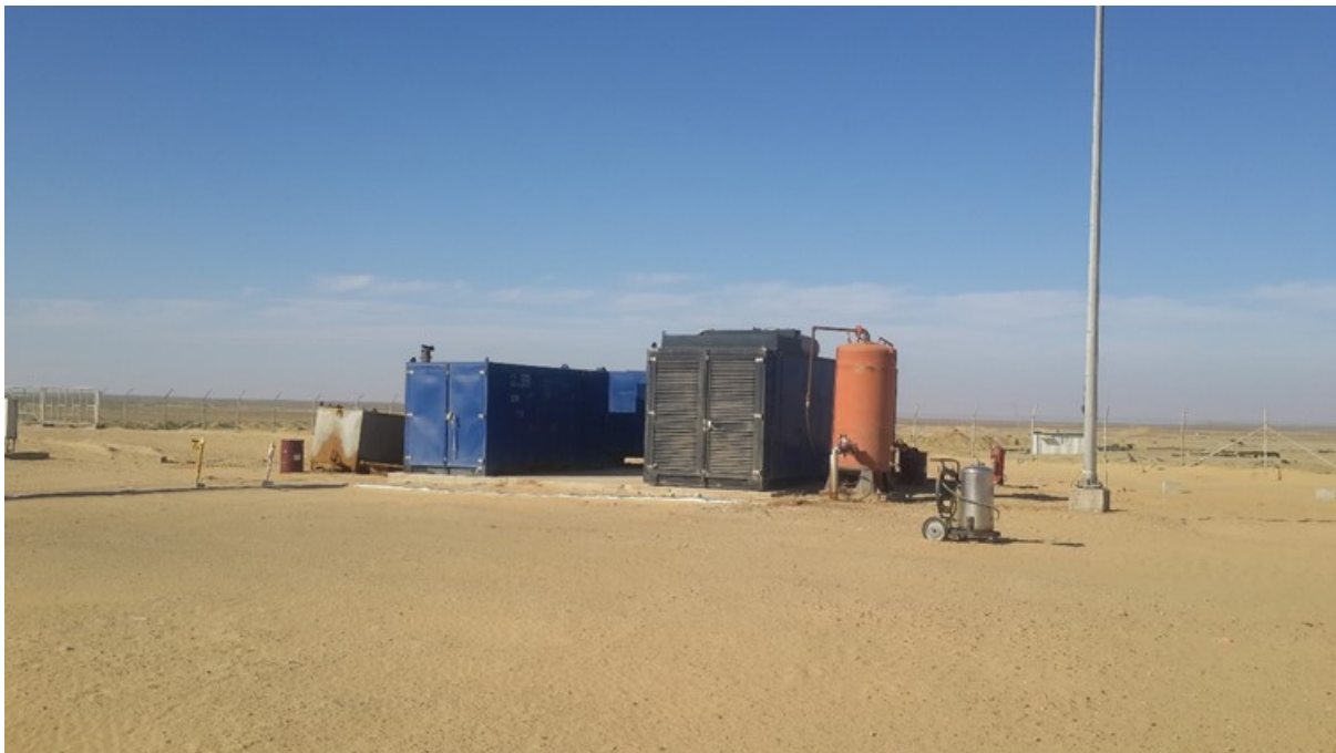
Figure AIV.7: Power Generators
