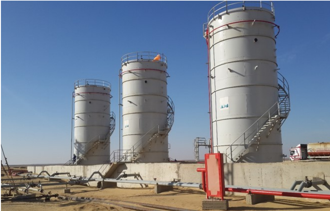
Figure AIV.1: Production Tanks at El Salmiya Oil Station
