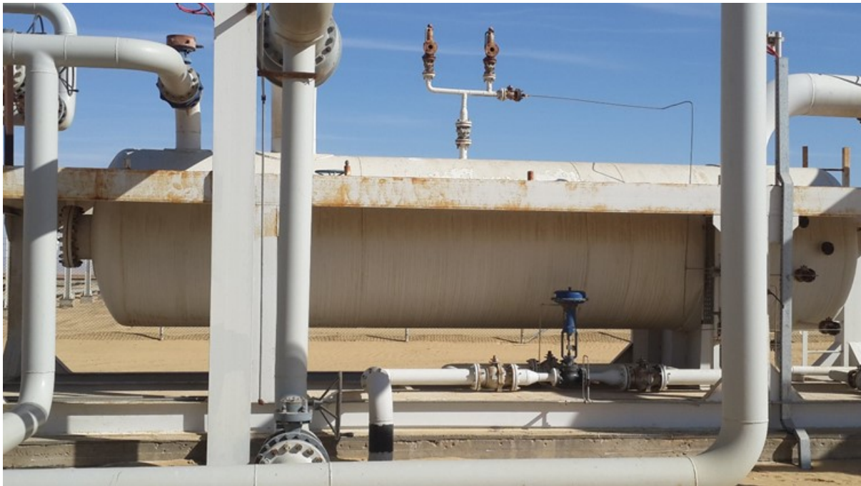
Figure AIV.6: FWKO Vessel and its Valves
