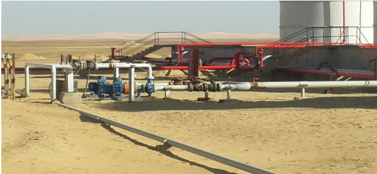
Figure AIV.4: Shipping Pumps at El Salmiya Oil Station
